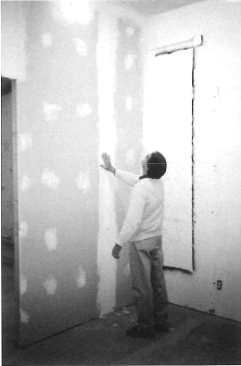
We've erected a wall in the back room to define the space. Here, Trustee and Project Manager Brian Dees is inspecting the construction work of Steve Butcher (who did the construction work in our other Museum space).
