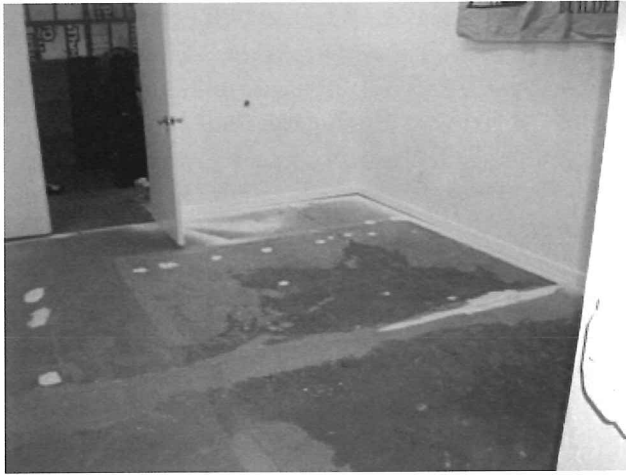
The work to make the 2005 expansion of space usable has been hard. Trustee Mark Brown had to strip the floor in a large room, and then lay down epoxy paint.
